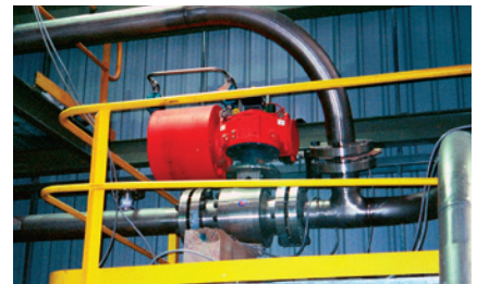
The highly corrosive atmosphere of autoclave vent valves is one of the industry's harshest and most punishing. This 6-inch 900 Class MOGAS valve has been in operation since 1999.
