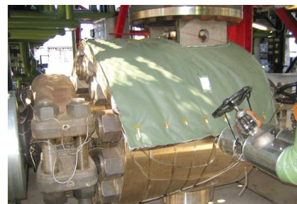
Located in a frigid Scandinavian environment, this large bore ASME 4500 class ball valve is installed on the outlets of the hydrogen heater.
