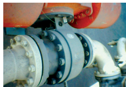
This CA-1AS 6-inch ASME 300 class feed isolation valve is a critical part of the emergency shutdown system.
