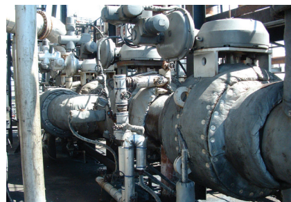
This midwestern refinery has four 20-inch ASME 300 class MOGAS ball valves in overhead vapor service. Several are in their second decade of service.
