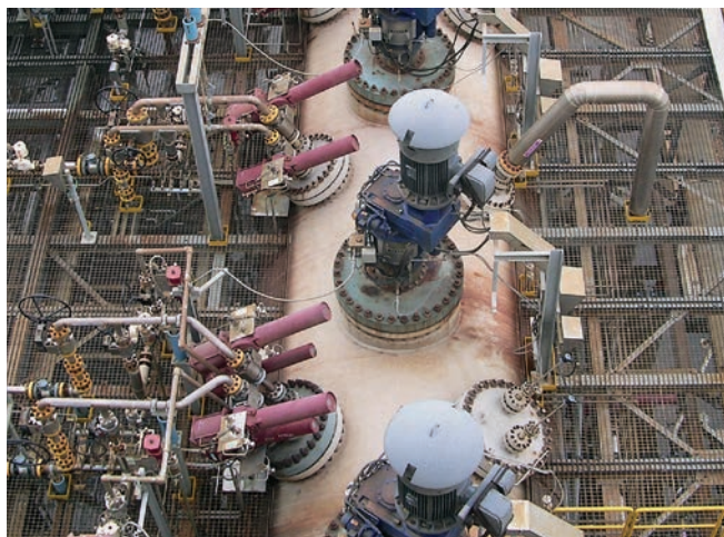
Large Asian mining complex maintains operational reliability in its autoclave utilizing MOGAS severe service ball valves. MOGAS' patented coating is a critical component to dependability of valve performance.
