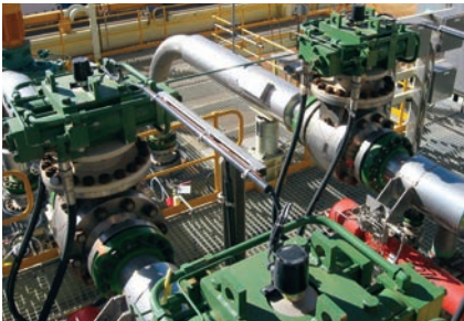
10-inch 600 class MOGAS valves with electrohydraulic actuators installed at a nickel HPAL operation.
