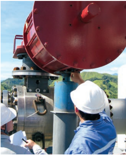
MOGAS field service technicians on-site during start-up of both autoclave plant and slurry transport pipeline at this remote location.
