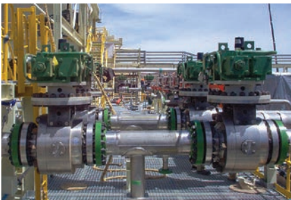
Multiple MOGAS valves were chosen with confidence to handle the punishing discharge system, one of the toughest applications in the operation.
