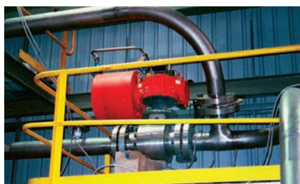
This 6-inch 900 class vent valve has been in operation since 1999.
