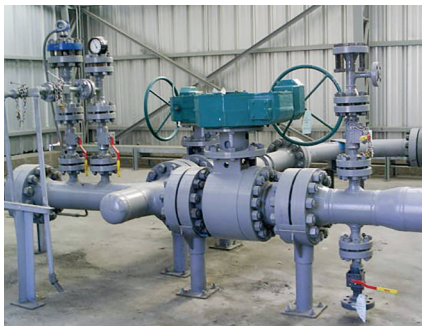
This hydrotransport pump station has 6-inch and 8-inch ASME 1500 Class MOGAS metal-seated ball valves, as well as numerous 2-inch ASME 1500 Class drain valves, which have all been operating since 1994.
