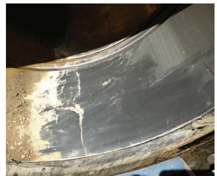
Under the same process conditions, the competitor's valve underperformed and required frequent maintenance due to erosion.
