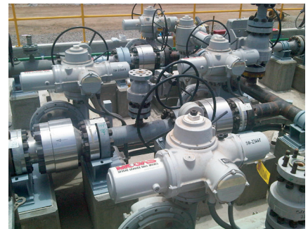
Absolute reliability for these CST-1, 6-inch isolation valves is very important due to the punishing effects of slurried ore, as well as being located 1,430 meters above sea level.
