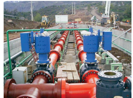
These 24-inch ASME 900 Class ball valves in a choke station have a stroke time of 45 seconds to handle copper concentrate with an average flow rate of 1167 liters / second.
