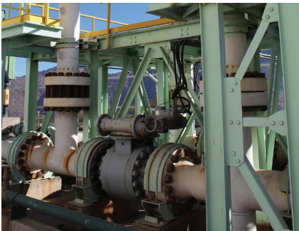
More than 120 C-Series valves, 2 to 24 inch, ASME 150-1500 Class, were installed on this concentrate line choke station to process copper slurry.
