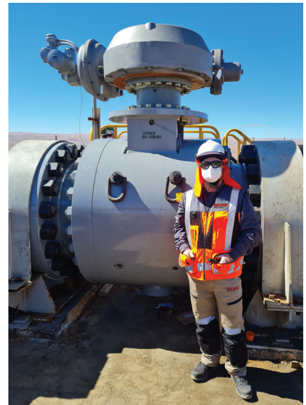
Four MOGAS T-Series (trunnion) 36-inch, ASME 900 Class valves are installed to support copper operations in the remote desert in Chile.
