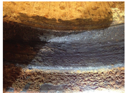
Material loss in the seat pocket was caused by galvanic corrosion, allowing leakage around the valve seats.
