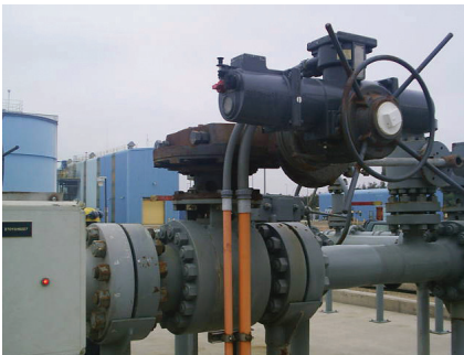
Multiple C-Series valves, 8-inch, ASME 1500 Class, cycle 28 times a month under differential pressures to successfully isolate copper slurry.
