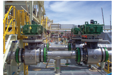
10-inch MOGAS valves / REXA electraulic actuators installed at a nickel HPAL operation.
