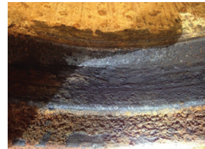
Material loss in the seat pocket was caused by galvanic corrosion, allowing leakage around the valve seats.
