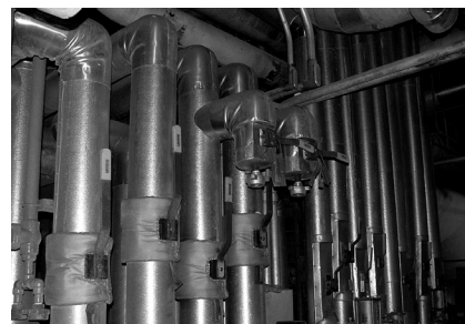
Wall of MOGAS RSVP valves for a main steam drain application have outperformed the originally installed globe valves. Exposed to 950°F at 1875 psi (510°C at 129 bar) while online, it is critical that these valves operate dependably.
