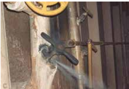
Continual stem leaks from globe valves decreases plant efficiency and causes maintenance costs to rise.
