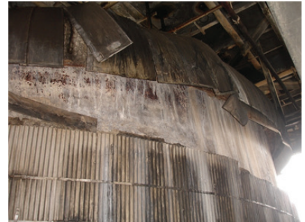
Leaking water from a competitor's valve caused damage to the coke drum's thermal insulation.
