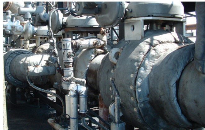
Four 20-in ASME 300 Class overhead vapor valves have been installed since 1991 at this refinery in Kansas, USA. After eight years of continuous service, less than 0.001 inch of the coating was worn away.
